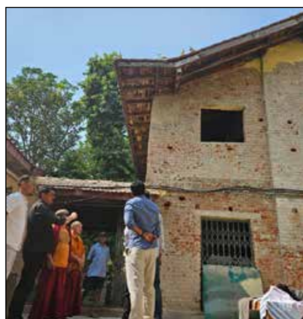
Chairman/CEC, LAHDC Leh, Tashi Gyalson visited Ladakh Buddhist Vihara in New Delhi to oversee the ongoing first phase of the renovation work funded under the Hill Council Leh's budget.
