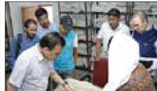
Commissioner/Secretary, Tourism & Culture, Ladakh, Kacho Mehboob Ali Khan reviewing the ongoing construction work of the Archives, Archaeology & Museums building at Skampari, Leh.
