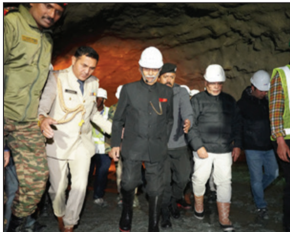
Lieutenant Governor of Ladakh, Brigadier (Dr) BD Mishra (Retd.) visited Zoji-La Pass and inspected the progress of the ongoing construction work on the Zoji-La Tunnel.
