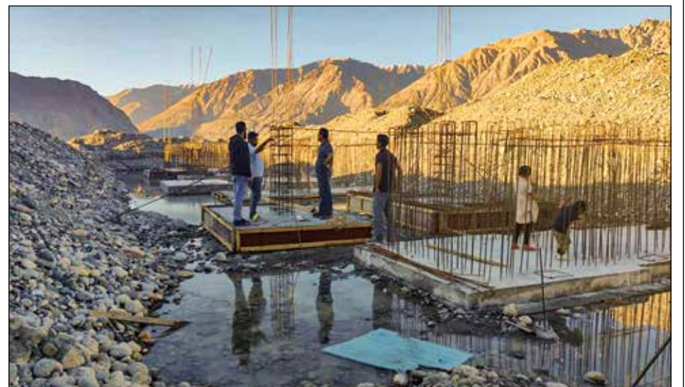
Deputy Chairman, LAHDC Leh, Tsering Angchuk visited the under construction 220/33 KV (GIS) Diskit Sub-station of the Northern Grid and took stock of the ongoing work progress.
