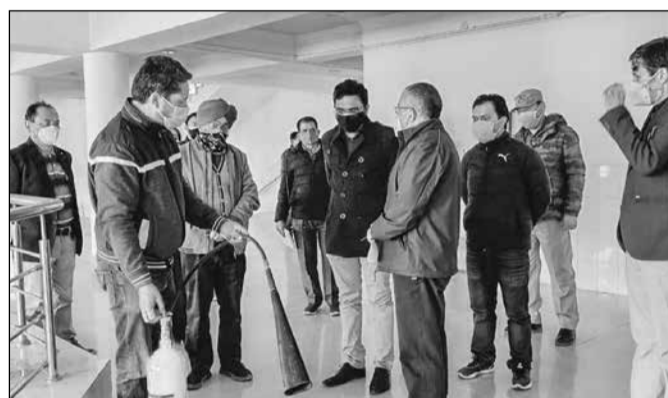
Chairman, DDMA Leh, Shrikant Balasaheb Suse inspecting the fire safety equipment installed at SNM hospital.
