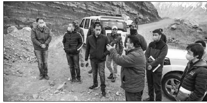
DC, Kargil, Santosh Sukhadeve along with officials taking stock of the pace of progress on the construction of lift irrigation system at Sodh area, Kargil.
