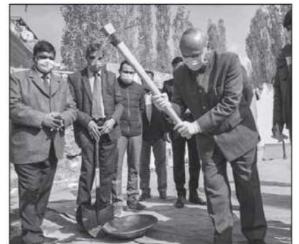
Lieutenant Governor R K Mathur laying the foundation stone for the construction of pre-engineered and prefabricated office block at Raj Niwas, Karzoo.
